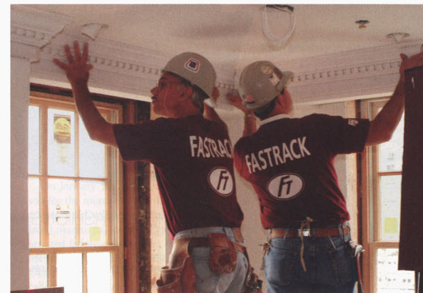
Fastrack Construction workers install dentil molding in the living room and dining room of the traditional flat.
